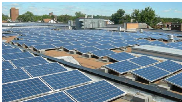
Above: PV array installation at Lord Stirling Community School in New Brunswick, New Jersey utilizing Solectria Renewables inverters
