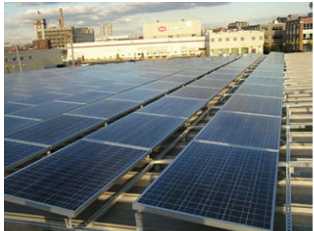
The PV array, located just off the I-93 in Charlestown, MA. This system utilizes a Solectria Renewables PVI 95kW grid-tied inverter and fused string combiners, with Evergreen panels. Photo courtesy of NexAmp, Inc.
